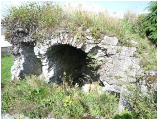
Fig.29: Before - Barrel vault to tower heavily colonised by plantlife.
