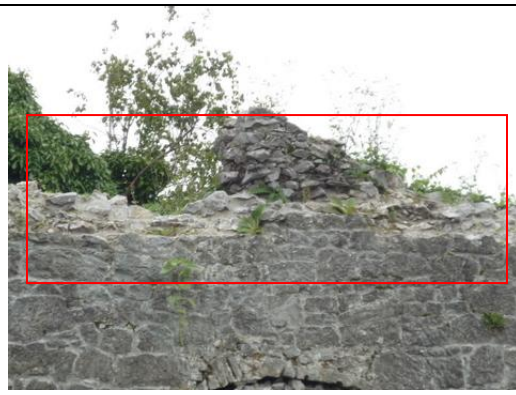
Fig.4: Failure of capping to Section D. Note the colonising of plantlife.
