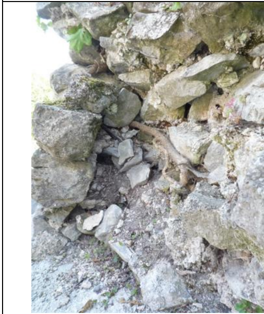
Fig.5: Exposed and loose rubble core to Section E of the Town Walls.
