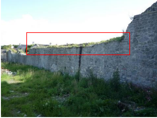
Fig.33: Before - Section D prior to removal of plantlife and failed capping at wall head level.
