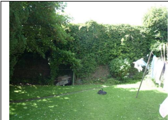
Fig.1: Significant plantlife and overgrowth to section A with associated open joints and areas of exposed core.
