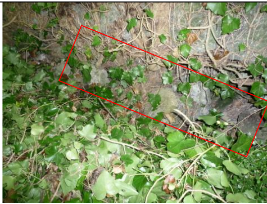
Fig.17: Before - Loss of stones at base level to section A.
