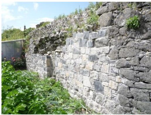
Fig.23: Before - Note the area of rebuild carried out during previous works c.2007.
