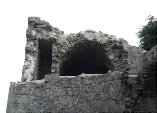
Fig.30: After - Barrel vault following removal of plantlife and flaunching of skyward surfaces.
