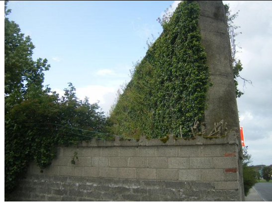
Fig.48: Heavy vegetation smothering the section of wall at the Mart Yard.
