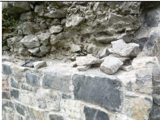
Fig.2: Erosion of the core and displaced stones at Section B.
